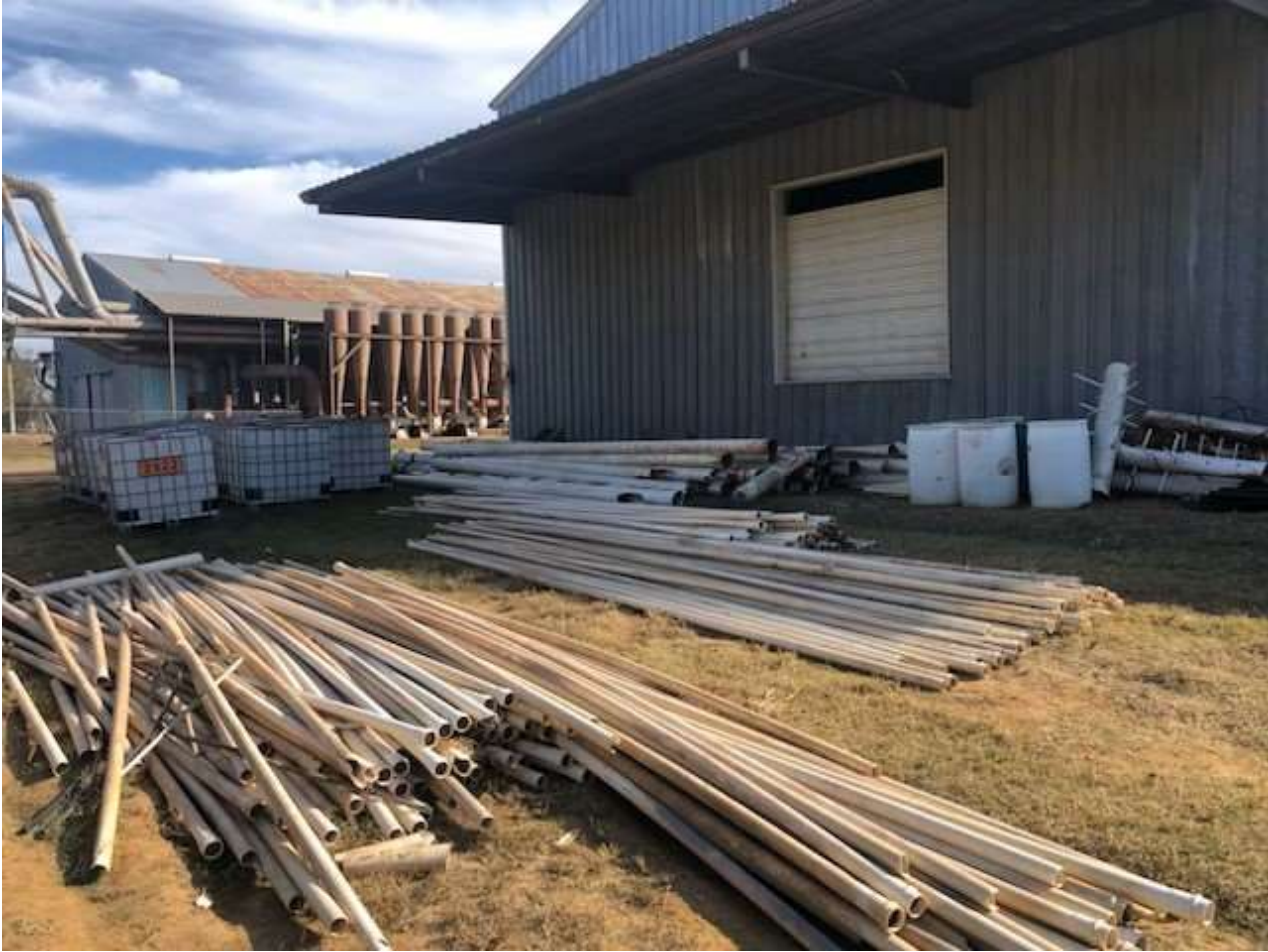
Attachment A. Donated PVC Pipe and Working Materials at Epstein Gin Worksite.
